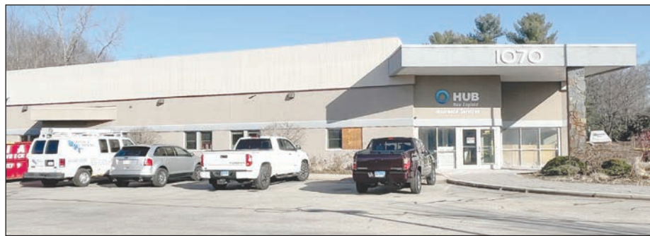
The interior demolition of the building is complete, now the construction team is working on building out. TURLEY PHOTOS BY QUINN SUOMALA
