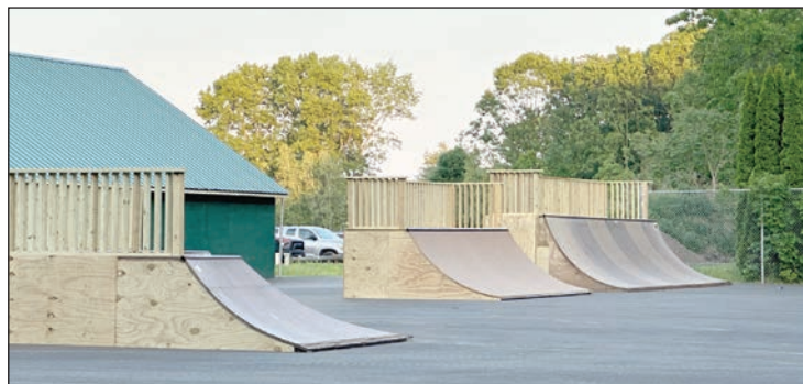
New ramps are constructed at the Agawam Skate Park. PHOTOS BY GREGORY A. SCIBELLI
