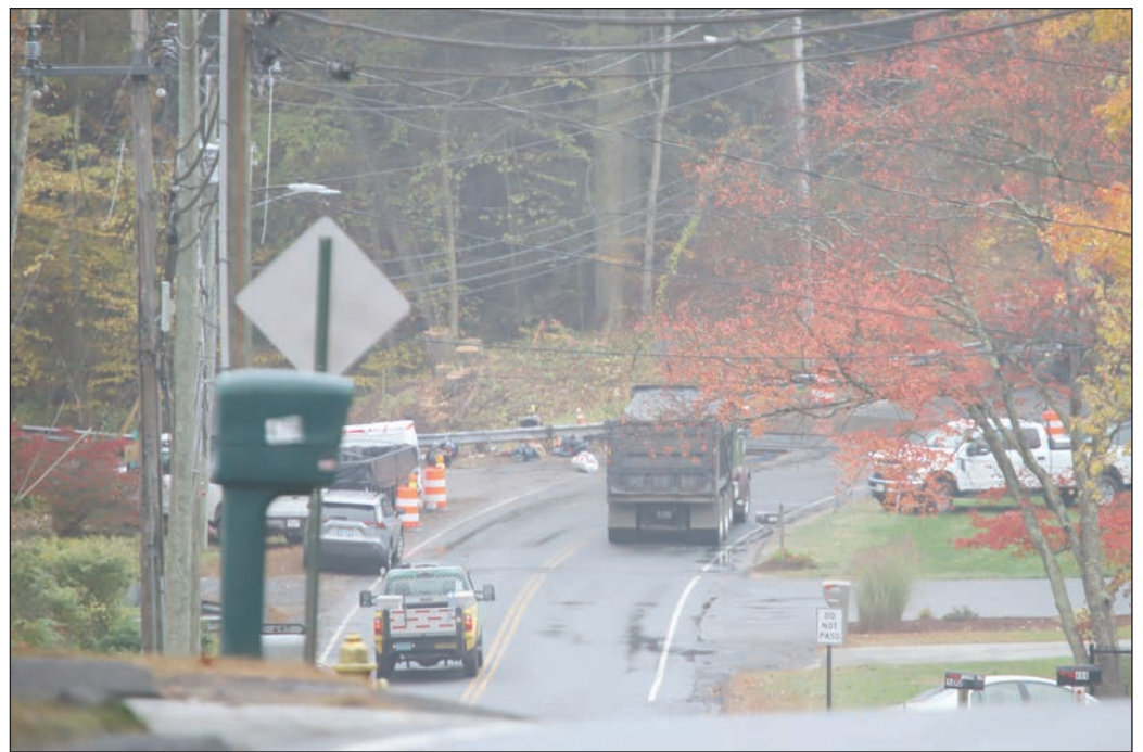
Crews get going on the initial work to repair a culvert on North St. last Friday. The repair work is projected to last until sometime December.
