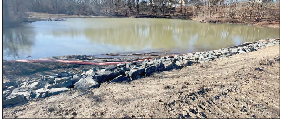
Upper Bemis Pond Dam will be removed as part of Phase III of the project to restore Abbey Brook.
