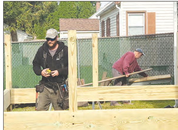
Volunteers work on repainting a back deck on 74 State St. during the Volunteer Service Day with Blue Cross Blue Shield and Revitalize CDC.
