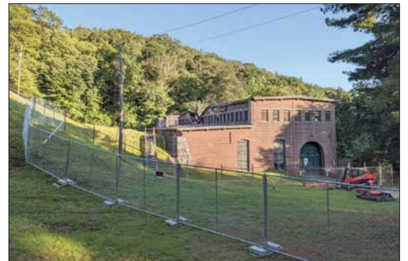
A full shot of the Red Bridge Hydro Plant on 5 Red Bridge Rd. which experienced a building collapse and small fire on Aug. 22.
