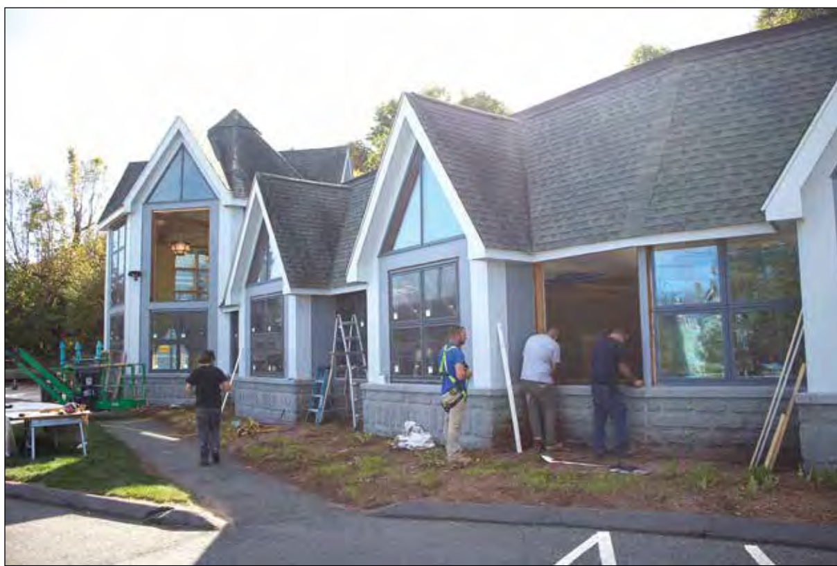
Turley Photo by Marcelo Gusmao Kolby Rodriguez, Nick Riley, Hunter Perron, Scott Theriault, and Caleb Duval have been hard at work repairing the windows at the Monson Free Library. After 30 years the library is currently undergoing window replacement.
