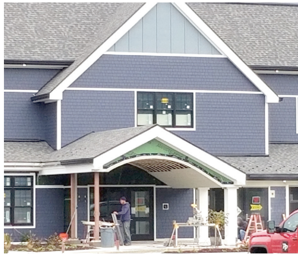
Our main entrance is taking shape! The area is covered by a portico to make access easier in inclement weather.
