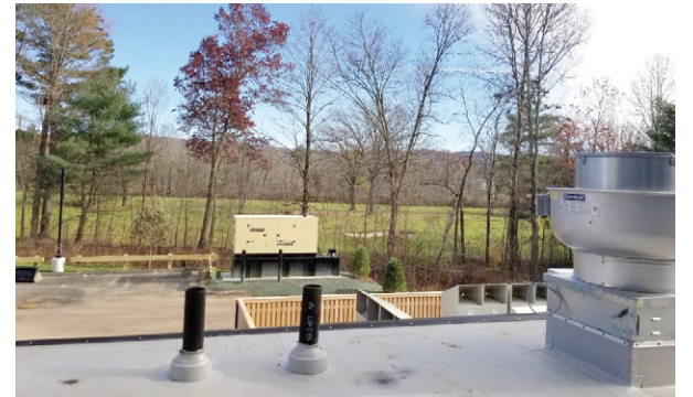
On the second floor, the view to the east shows a County Club fairway. In the near distance is the emergency generator for the Senior Center that has yet to be placed in its permanent home.
