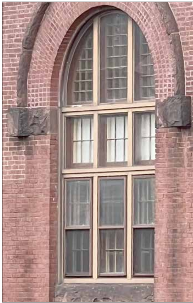
Submitted Photo This is one of the Town Hall windows the Friends of Ware Town Hall are working to restore.
