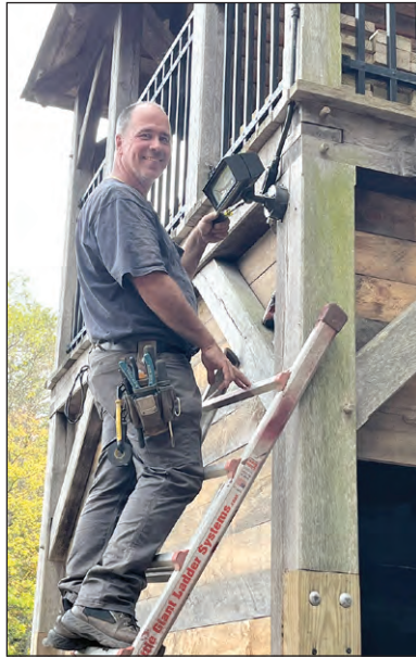
Bill Tinker of Hardwick, master electrician, volunteered to make repairs to electrical wiring and installed floodlights outside and lights inside the gazebo at New Furnace Landing, part of Ware River Park in Gilbertville.
